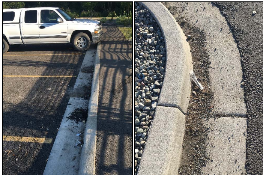
Dirt and Debris on the Porous Asphalt and in the Gutters
